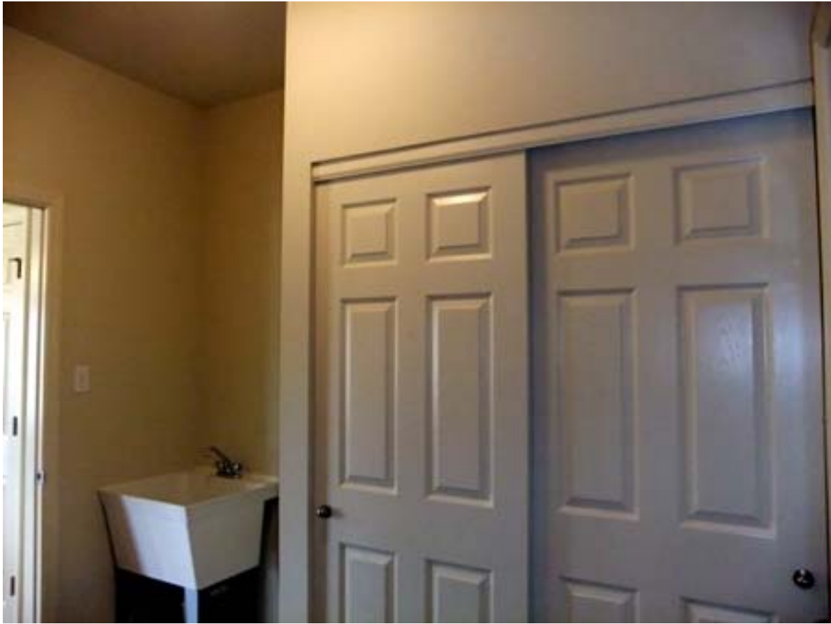
1 ST FLOOR LAUNDRY
